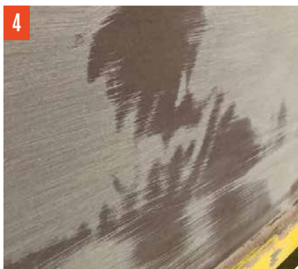
Areas not hit by the sanding block remained dark and shiny. FIG. 4
