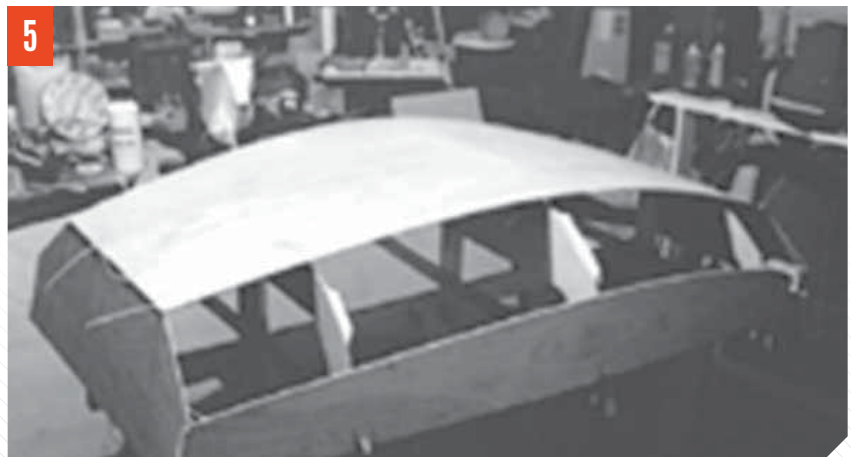
HARD CHINE PLYWOOD/STITCH AND GLUE Popular for first time builds for the ease of construction. Panels are stitched together over top of a frame to hold shape until joints are reinforced. Showing construction of a pram.
