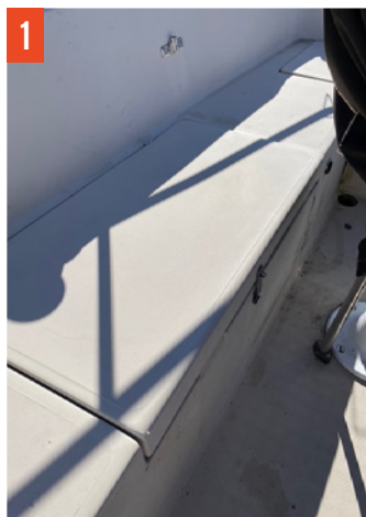
The lazarette was spongy. The top delaminated from the core.
