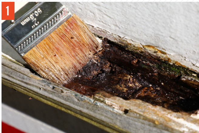
1 Coating rotted wood on a spray rail with Wood Rot Repair Epoxy.
