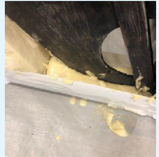
Shrink wrap tape is used to contain the foam into the open cavity.
