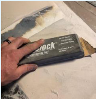
Sanding block is used to remove any epoxy that is higher than the fiberglass laminate.
