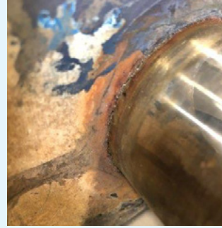
Crack around shaft is an indication of water intrusion.
