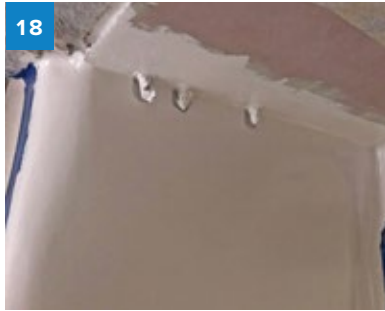
The surface was painted with flat white paint to finish the repair.
