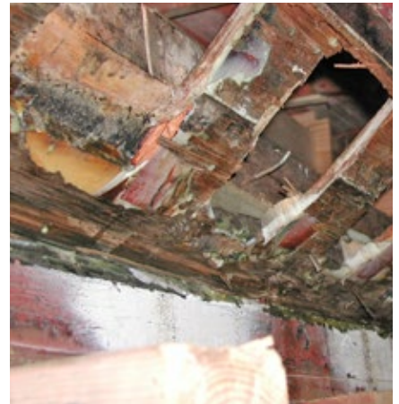
We shored up the boat under the hull for support. Initially, we removed the garboard, first, and second strake planks before starting the first stage of the rib repair. Using a chainsaw, we cut out the keel in 2' sections, and then installed a plywood mock-up of the new keel.
