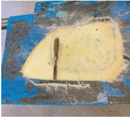
Fiberglass removed from a section of the rudder.
