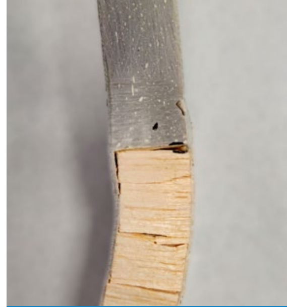
Close-up of the epoxy filled repair. Its fiberglass and balsa core fractured right at the transition from epoxy to balsa core.
