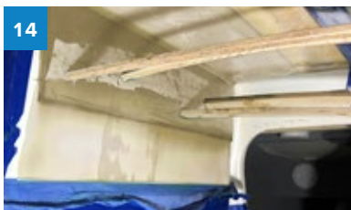
14 The G-10 panel bonded to the underside of the deck and the 1/4" thick fiberglass panel bonded to the daggerboard case. Prop sticks helped to hold the panel into position until the Six10 cured.
