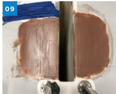
09 WEST SYSTEM 105/206 thickened with 407 Low-Density filler was used to fair the repair with the existing deck.
