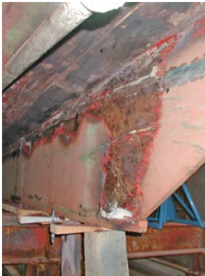
1989 keel check with epoxy repairs still good.
