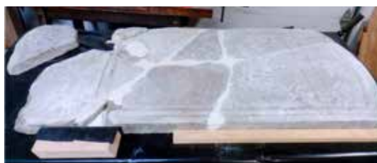
The cleaned pieces of headstones midway through assembly. Pulverized marble and white pigment mixed with epoxy helps the joint color match the headstone.
