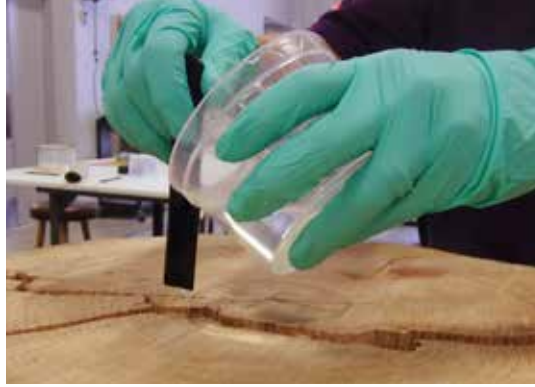
Pouring epoxy onto a mixing stick directs the epoxy into the bottom of the cavity.
