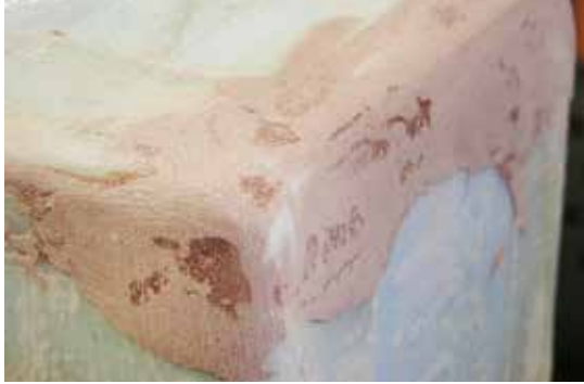
After glassing, the edges of the box were coated with 105/206 and 407 filler then faired.
