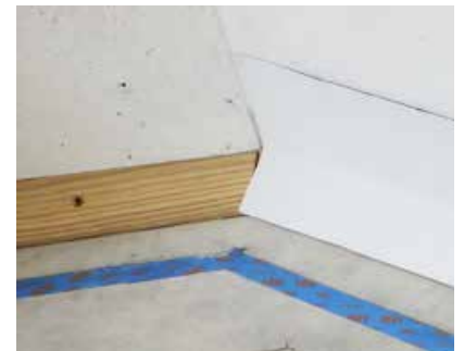
The wood strip on the left is a 45° beveled piece ripped from "two by" PT lumber. The right is six inch wide "peel and stick" flashing membrane.
