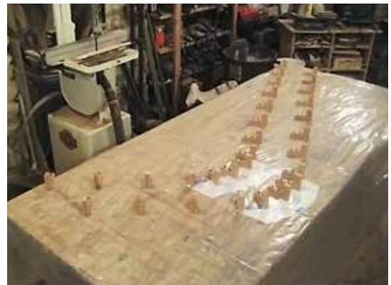
The crane's legs lofted onto a plywood workbench with poly sheeting and brackets for clamping the laminates.
