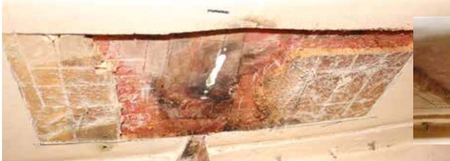
The rotted and wet core removed.
