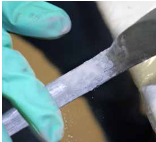
Brushing the repair site with aluminum powder to match the texture of the surrounding surfaces.
