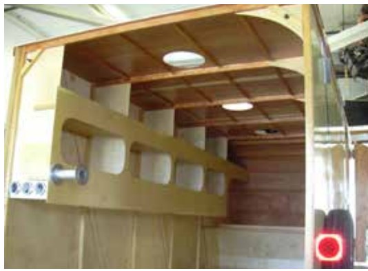
Three 12" diameter holes were cut into the top as skylights made out of polycarbonate.
