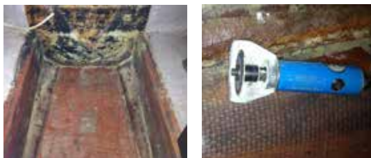
Left—The cabin sole with a layer of chopped strand mat Right—Rotary cutting tool for cutting through the chopped mat tabbing
