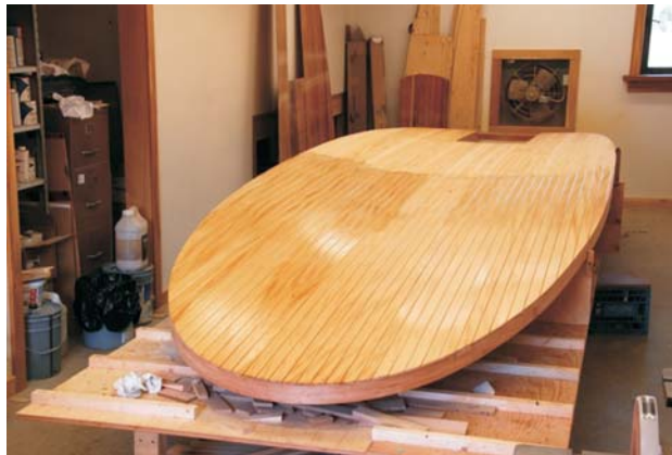
The underside of Sparks' cabin top is a basswood veneer applied in a traditional ceiling pattern. Working overhead is never pleasant so we finished it before installing. The basswood was very thirsty and absorbed enough to make a dense, stable base for varnish. A second coat was applied, rubbed in and wiped off to create a glossy surface. The scuffing pad was the ideal tool for this step as it fit into the cracks between the planks and worked the groove into a smooth, repeatable shape. Excess epoxy in the crack was picked up by the pad, preventing flooded joints.
