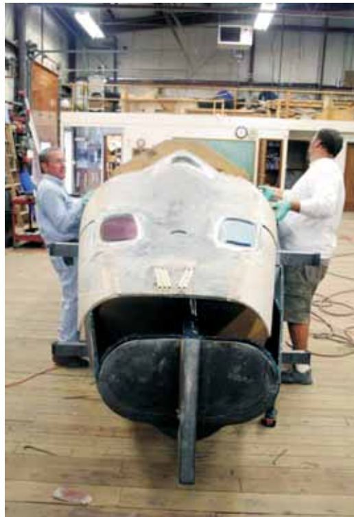
Left—Jan applies thickened epoxy adhesive to the tops of the bulkheads and side fuselage skins before the deck is installed. The main bulkheads were \frac{1}{8} " plywood over 1" foam with interior wood trusses, covered with carbon fiber skins. Heavy bulkheads have an additional three layers of carbon on each side.
