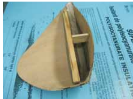
Two plywood panels are joined over a temporary form to produce the desired shape.
