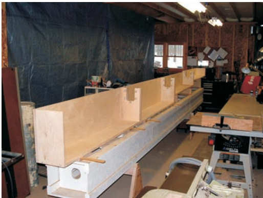
Dry fitting the tanks in the shop. The tanks are built of 1"-thick, 16-ply birch-faced plywood.
