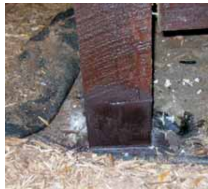
Blackmon finished the repair with a coat of dull brown paint to camouflage the epoxy base.
