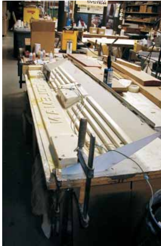
The grill is clamped to remove twist while the repairs are made and the epoxy cures.
