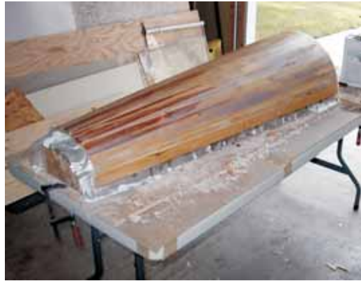
Left—Tapered \frac{3}{8} " thick strips are tacked to the mold. The gaps were then filled with epoxy thickened with 410 Microlight.
