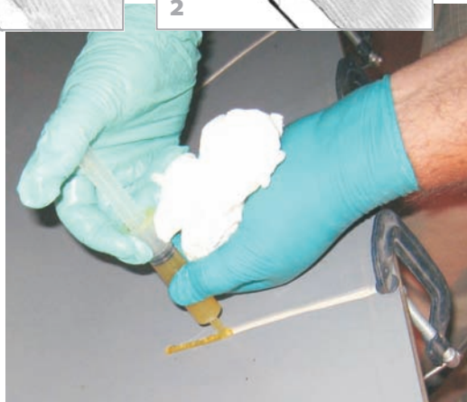
Injecting G/flex into a widened crack. Note paper towel in hand to clean up after rampant sloppiness.
