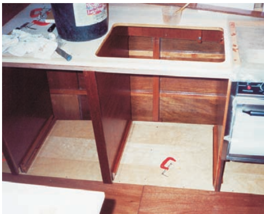
The galley under construction. Throughout 2004 work continued on the interior cabinetry and building of the fuel, water and waste tanks.
