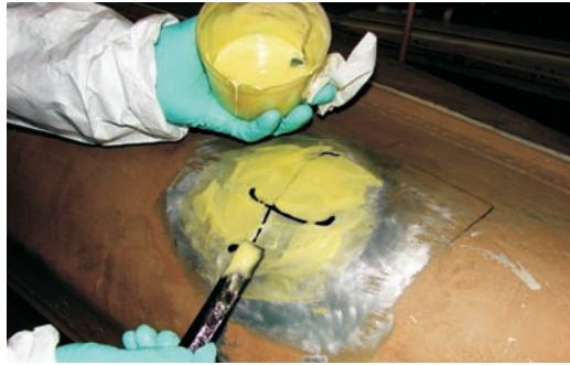
Photo 4 —Left, 12 oz fiberglass patches for both the inside and outside were wet out with G/flex 650.
