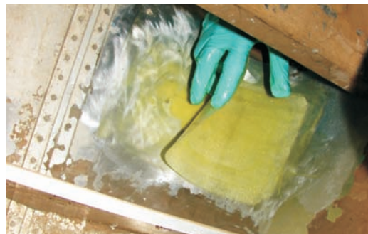
Photo 7 —Three layers of glass were laid in position on the inside of the hull and lightly squeegeed to remove trapped air.
